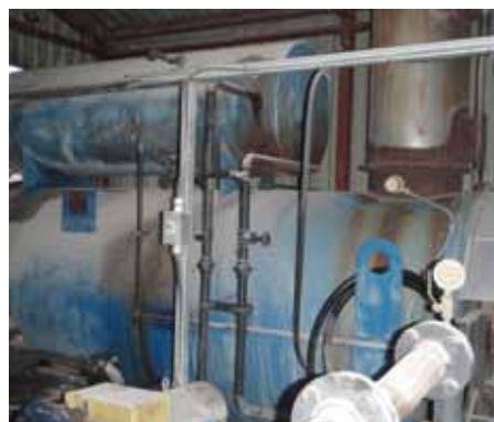
Hot Oil Heater
