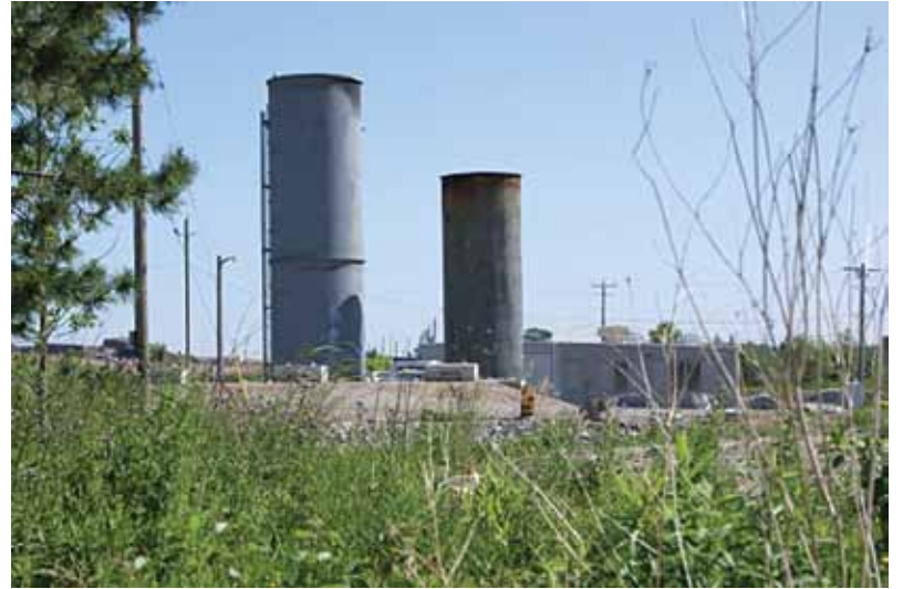
The two enclosed flares at the WEGI East & South Landfill Gas Plant, Niagara Falls, ON.
