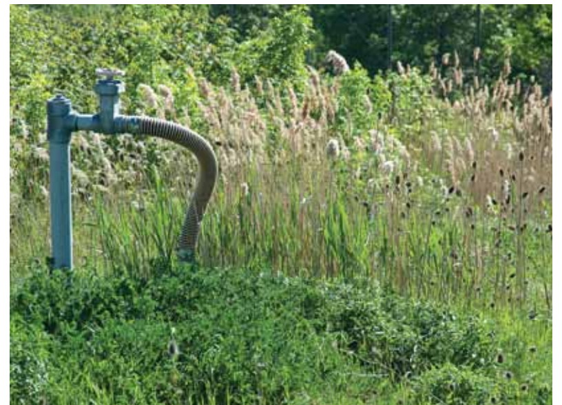
Landfill Gas Extraction Well
