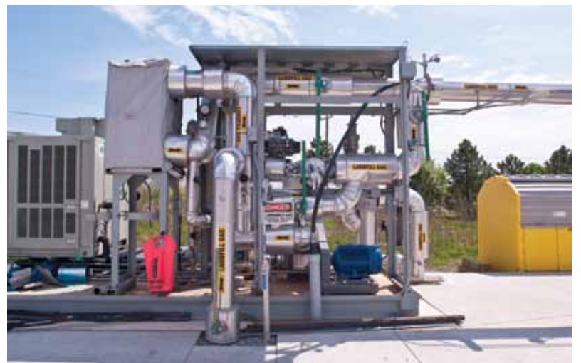
Landfill Gas Compression and Treatment
