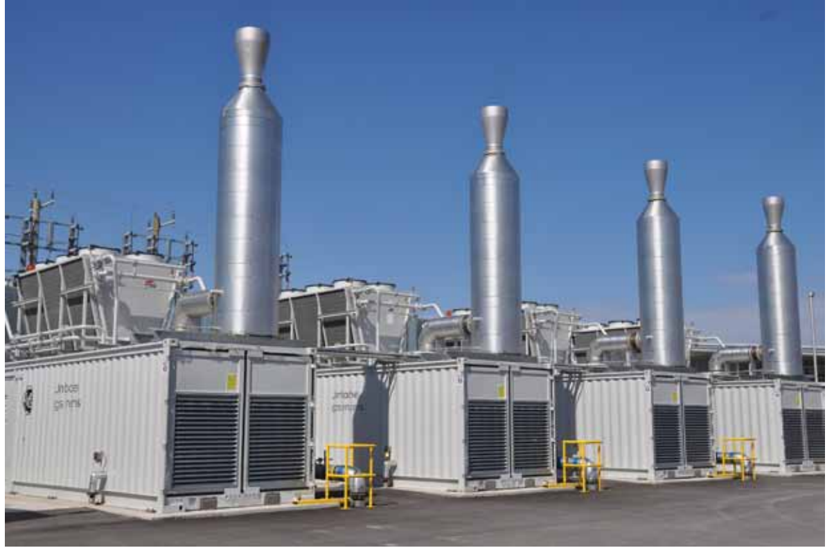
Moose Creek Energy Plant, Ottawa, ON
