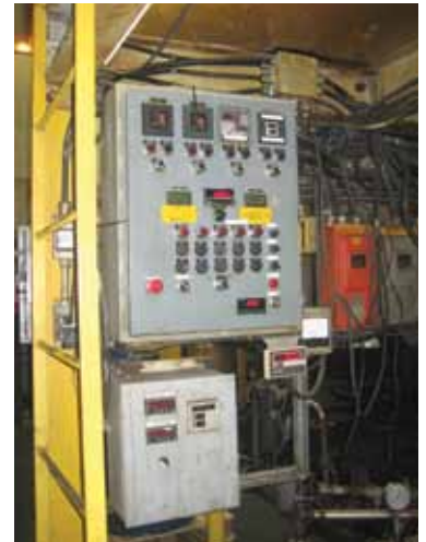
Solution Control Panel
